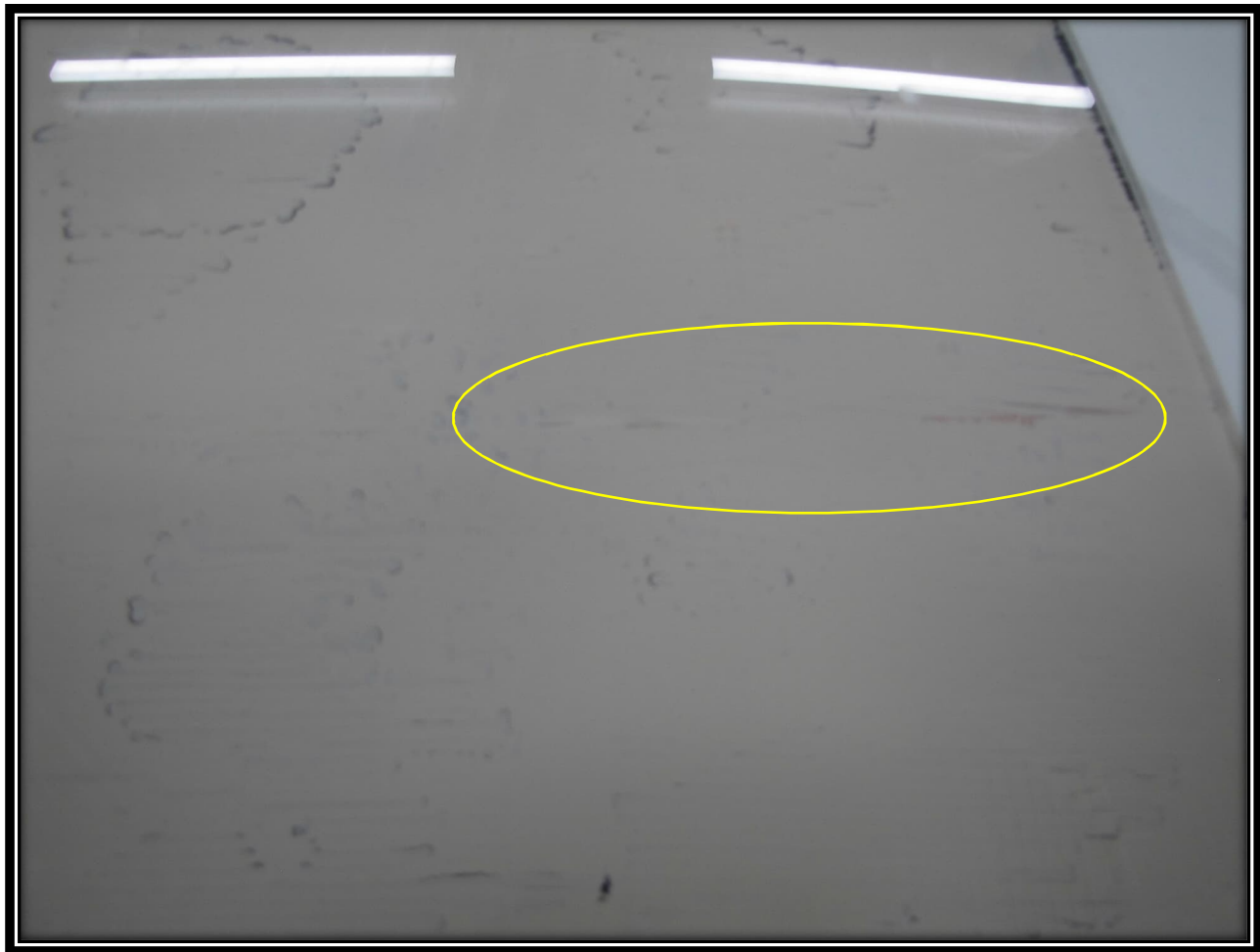
Water penetrated to the Perspex base along the joints.
