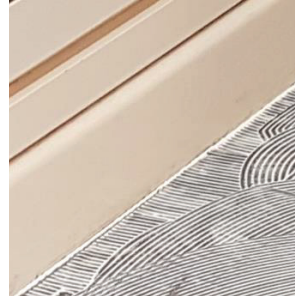
Silicone to the shower/ floor junction
